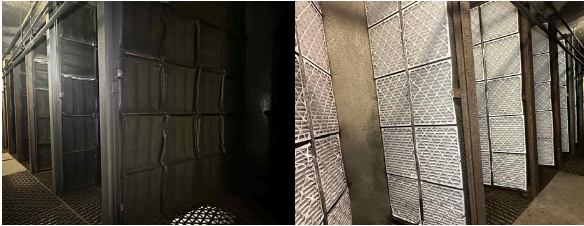
Latimer Hall Mechanical Room Before and After Air Filter Replacements
