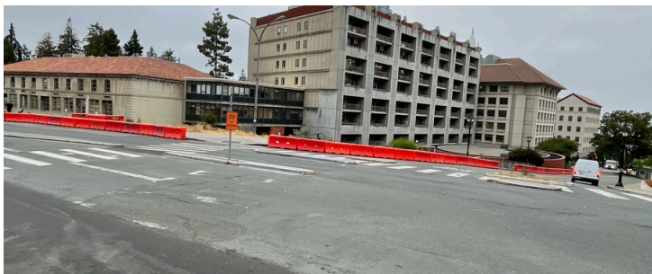
Water barricades at Gayley Road and University Drive NOTE - Water barricade toppers with privacy screen to be installed week of 07/08 - 07/12
